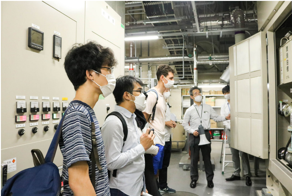
Participants observing the insides of a core electricity generator of Hokkaido Gas Company.
